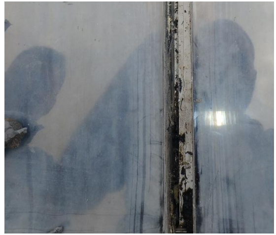
Photo #02 Sealant removed from vertical joint.
