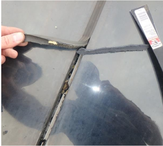
Photo #01 Sealant removed from vertical joint.
