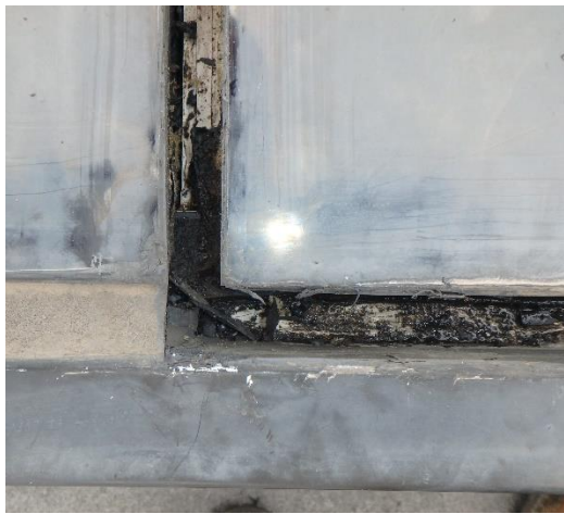
Photo #03 Sealant removed at vertical to horizontal joint intersection.
